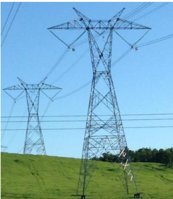
Figure D.27: Western Alberta 500 kV transmission line
