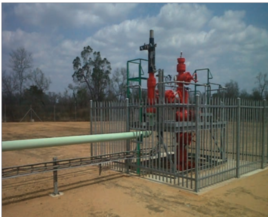
Fig 1 - Remote monitoring equipment
