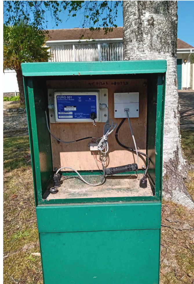
Pressure management and control data logger - communicates status at the extremities of the gas network to inform usage models.
