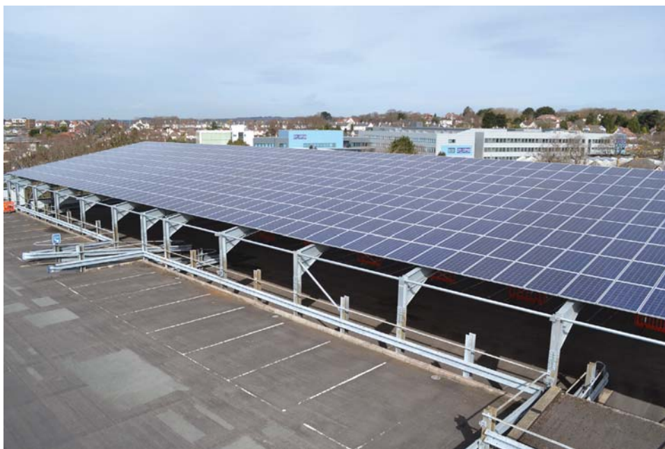
▼ Figure 3 Solar arrays on the roof of the multi-storey car park
