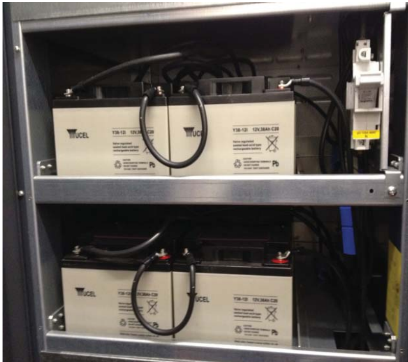
▼ Figure 3 Example battery ELV supply
